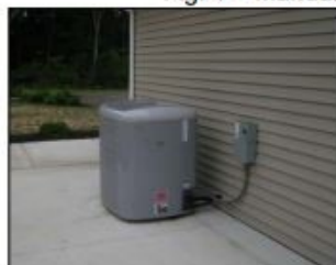
Fig. 2 – High-Efficiency Carrier split system
